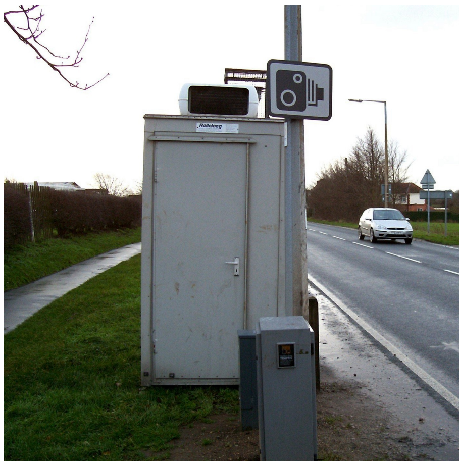
Figure 26.1 Real Time Air Quality Monitoring Station in the East Riding
