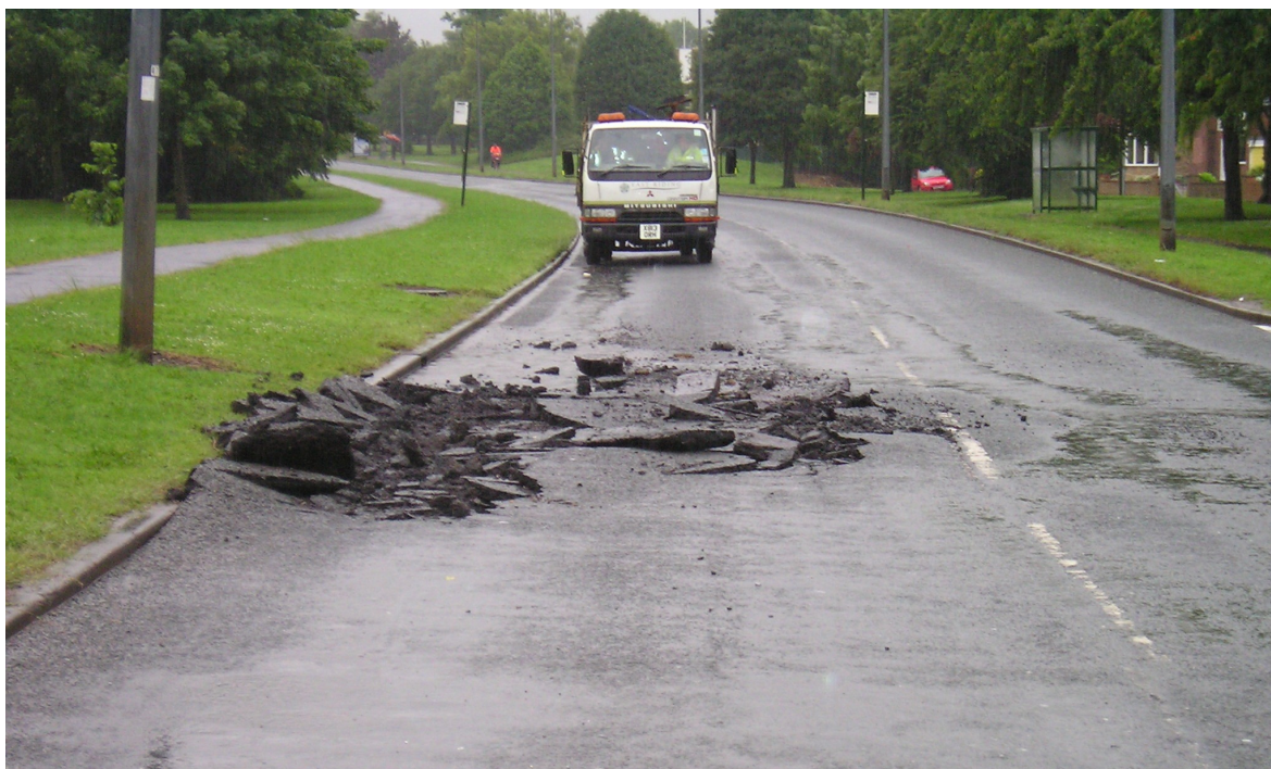
Figure 14.1 Flood Damage to the Highway in Anlaby (2007)
