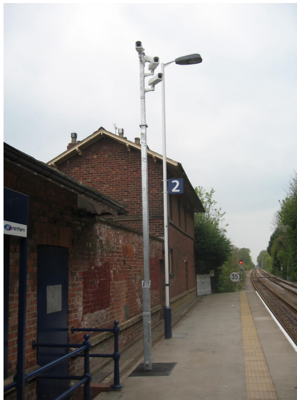
Figure 18.5 CCTV at Cottingham Rail Station
